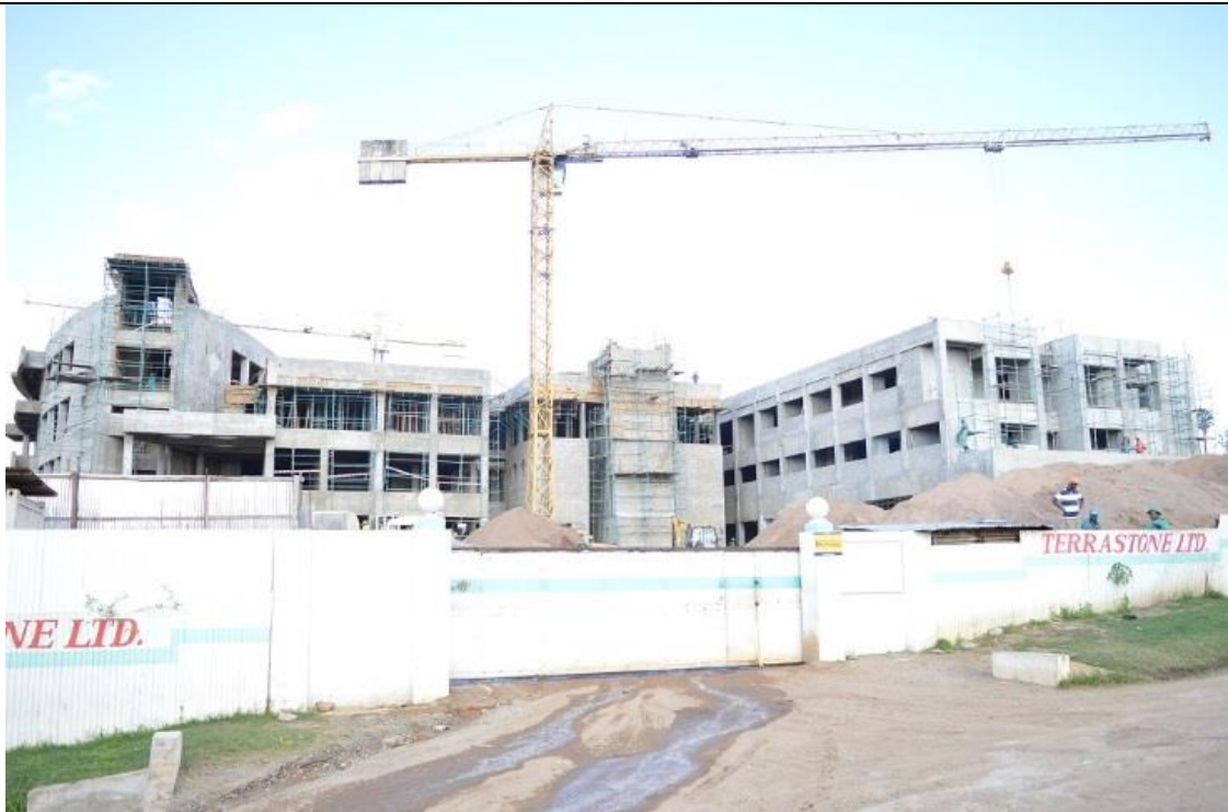
Photo of the front of the new MBS laboratory complex under construction in Blantyre
