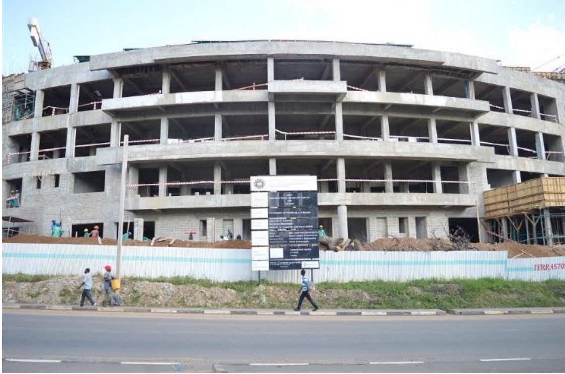
Photo of the front of the administration block for the new MBS laboratory complex under construction
